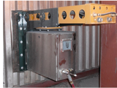
Valmet Furnace IR Camera Installation
